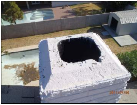
Photo: Chimney cap defects include cracks and holes and missing rain cap/pest cage.
